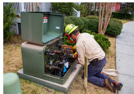
The cost for a typical pad mount transformer has doubled in the last two years
